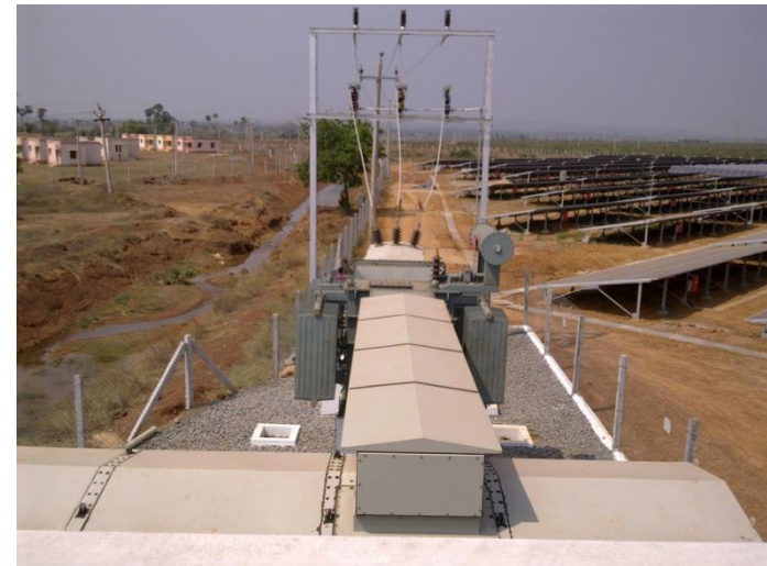
Substation at Power Plant
