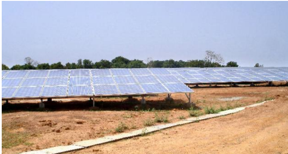
Evacuation of Power Solar Farm
