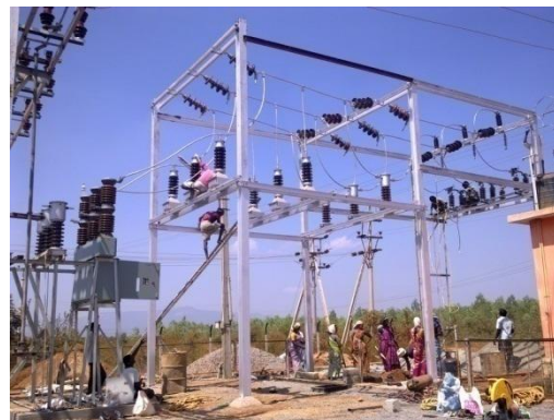
Bay extension at DISCOM Substation
